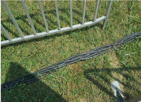
This fence was found against these wires.
