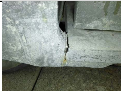
Large Crack in Caster
